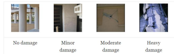
Fig. 7. Damage level detection: no / minor / moderate / heavy damage.
