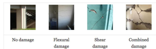
Fig. 8. Classification of: no / flexural / shear / combined damage.
